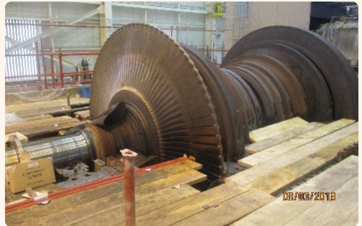
LP Turbine Inspection 2019
